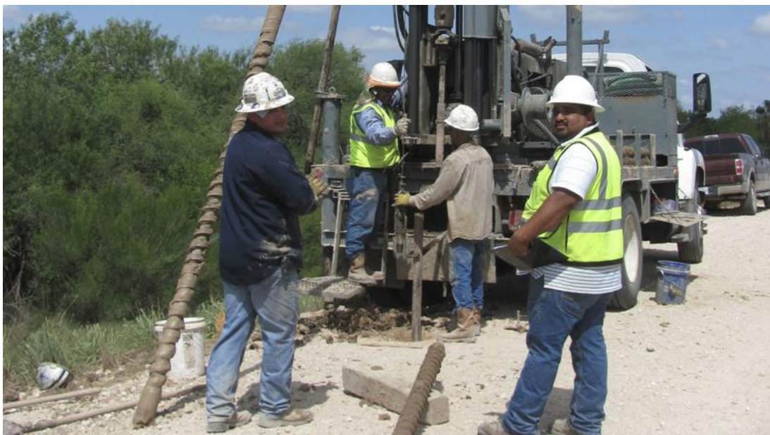
A crew uses a drilling rig to extract soil samples in the Santa Ana National Wildlife Refuge in Texas. (Jim Chapman / For The Times)
