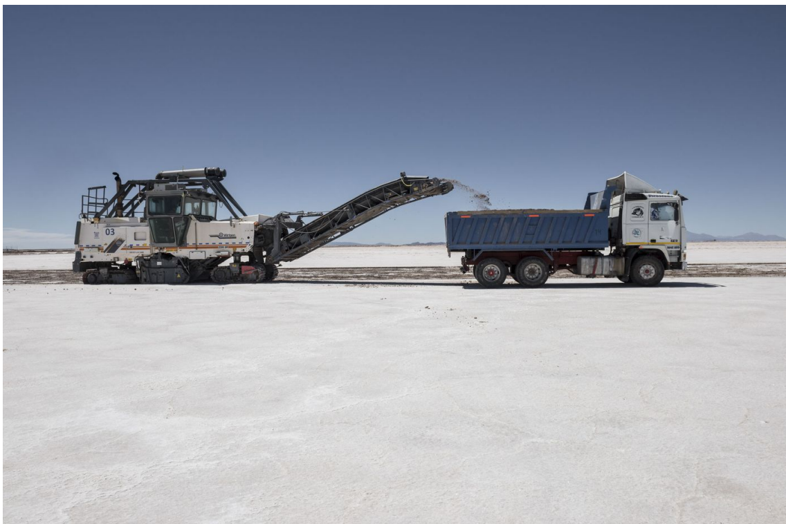
A machine loads soil into a truck during the construction at the Uyuni salt flat in Bolivia.
