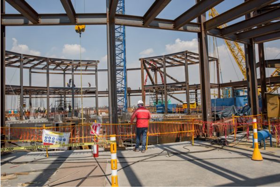
Construction at the New International Airport of Mexico City (NAICM) in Texcoco, in April 2018.
